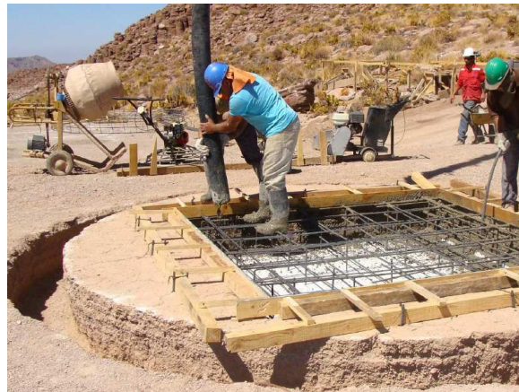
Figure 21. Pouring concrete for a 1-meter LCOGTnet telescope at the Cerro Tololo Inter-American Observatory in Chile.
